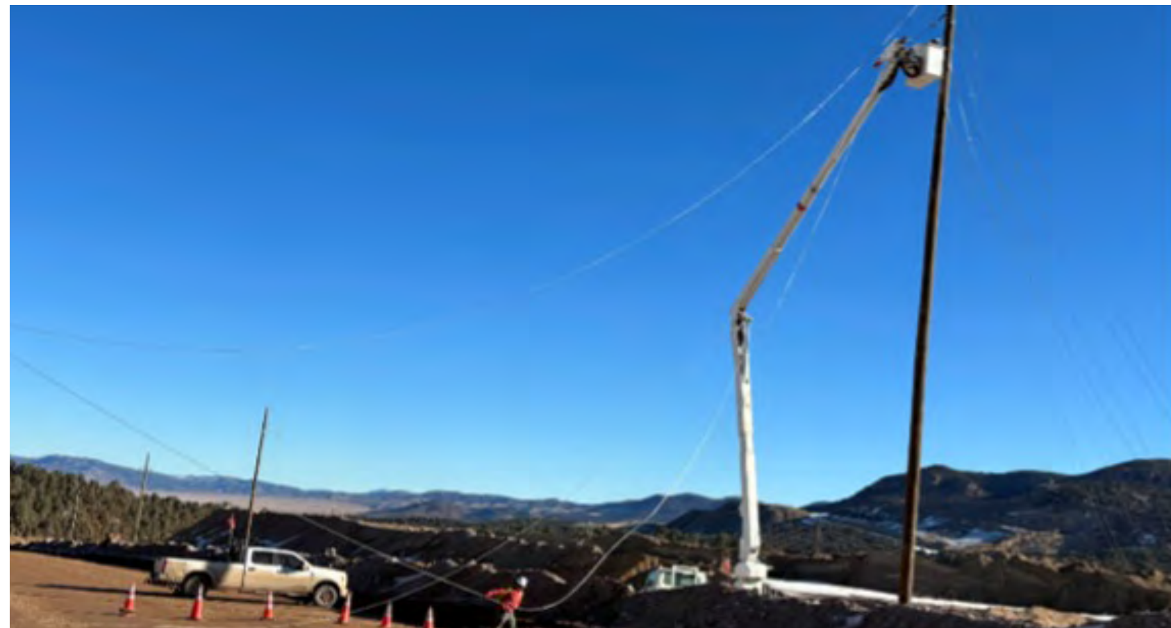
At Bald Mountain, access to grid-connected line power.
